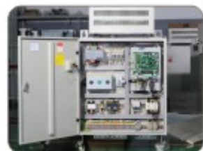
控制柜Control Cabinet
